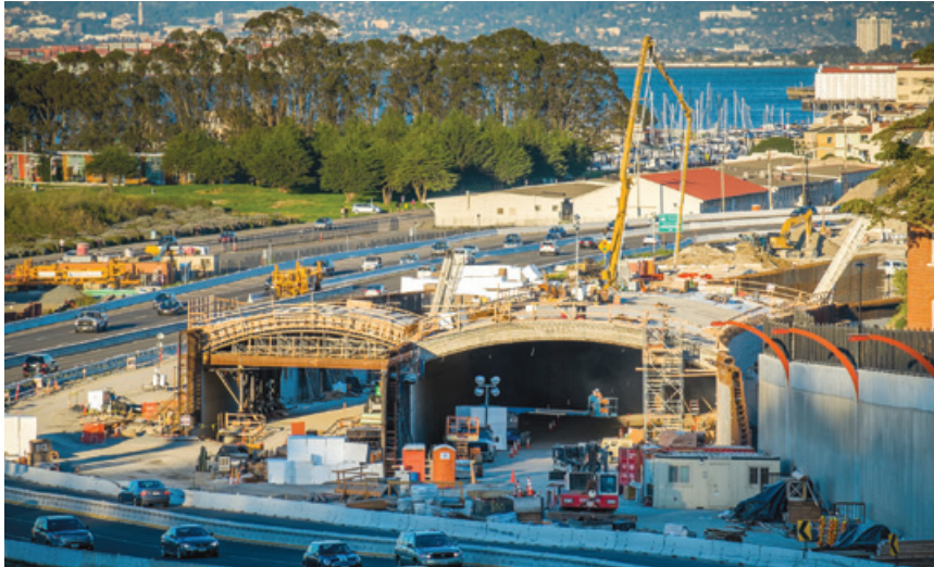
PARTNERSHIP CH2M Hill did the design work on the Presidio Parkway, a P3 project in California.
