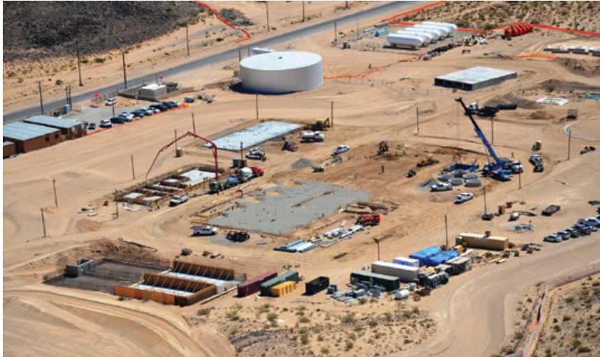
POPULAR APPROACH A treatment plant in California is one of several design-build projects underway.
